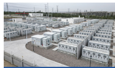
Standalone BESS Project Ningxia 100MW/200MWh
