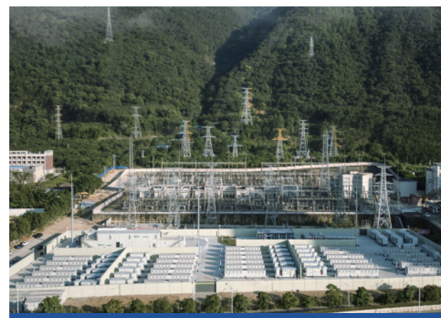
High Temp./Humidity, First Commercially Operated Grid-side Standalone BESS Guangdong 100MW/200MWh
