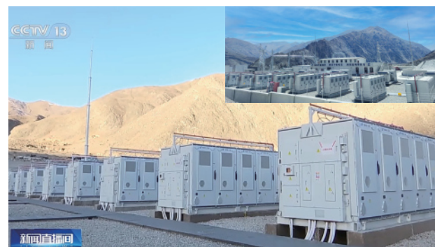
World's Highest Altitude (5,100m), Extreme Cold Energy Storage Power Plant, Southwest, China 10MW/40MWh
