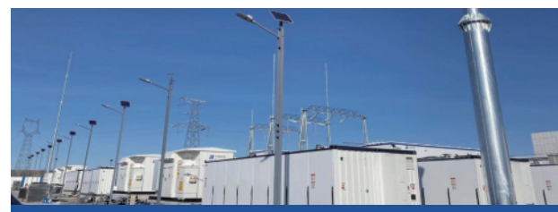
First Extreme Cold BESS Project Inner Mongolia, China 60MW/120MWh
