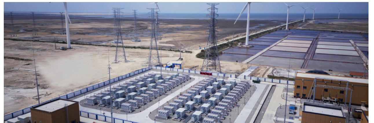
High Temp./Humidity/Salt Fog Wind + BESS Project Shandong 100MW/200MWh
