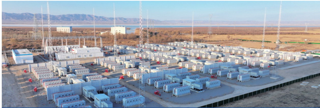
The Largest New Engery + BESS Project in 2023 Northwest, China 300MW/1,200MWh
